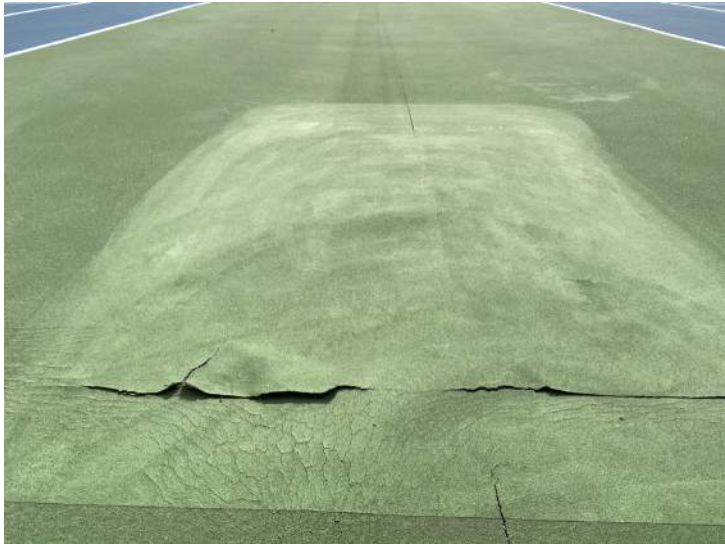
TENNIS COURT CRACKS
