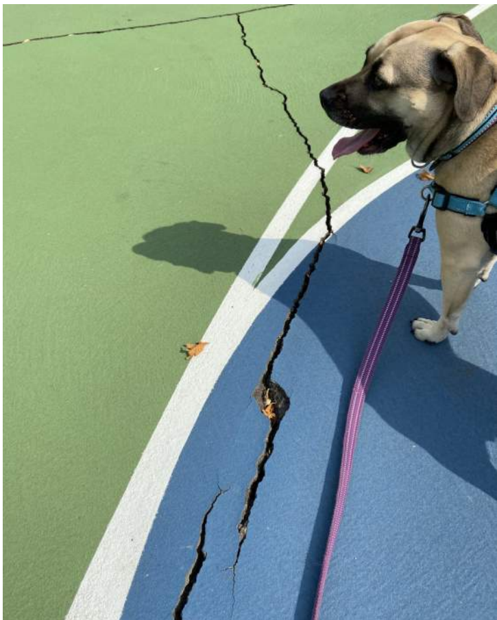
BASKETBALL COURT CRACKS
