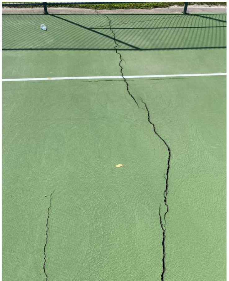
TENNIS COURT CRACKS
