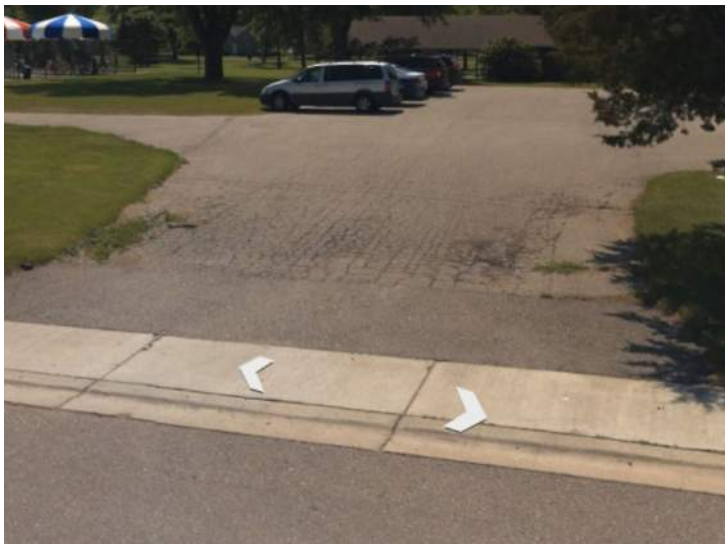
PARKING LOT CRACKS
