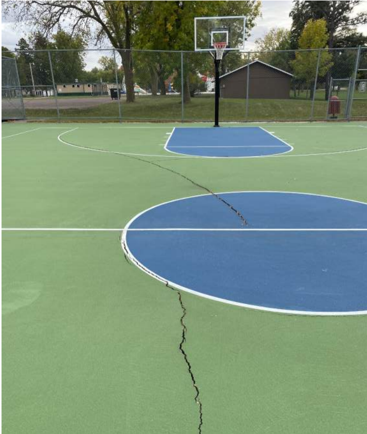
BASKETBALL COURT CRACKS
